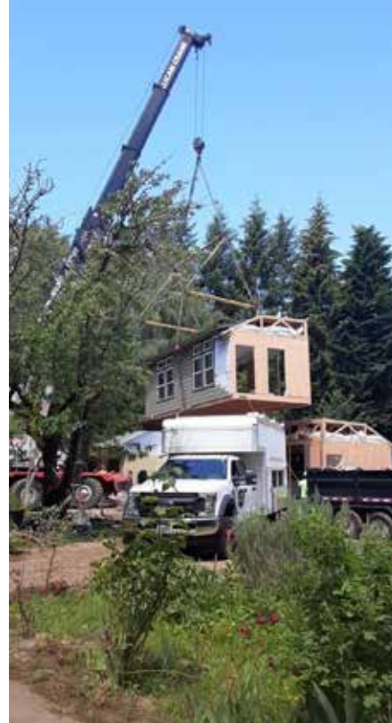
A modular project in-progress in Normandy Park shows a new method of residential building.
